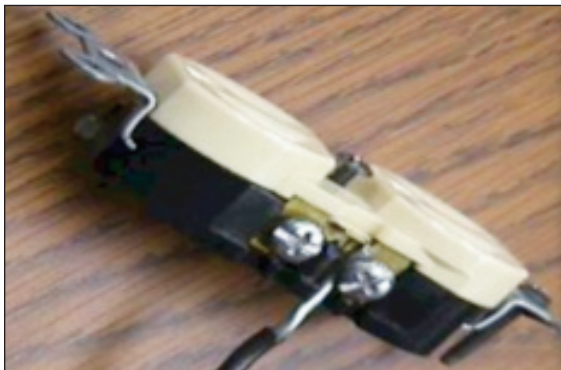
Aluminum wiring was prevalent in the 1960s and 1970s.
