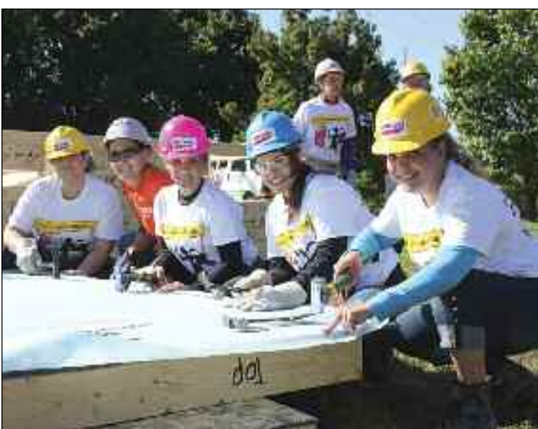
Women work on the Brimley Road site in 2014. The diocese will have four days this year in which to send teams to help with construction. PHOTO BY HABITAT FOR HUMANITY GTA
